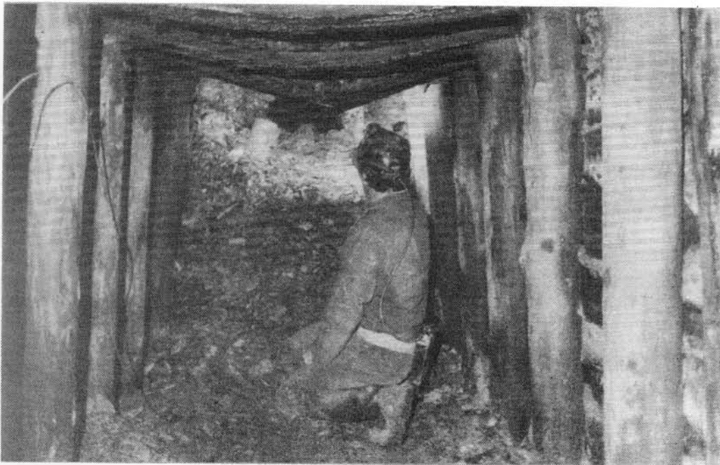
(4) The collapsed roof and timbers near the end of the accessible part of the incline in 1984.
