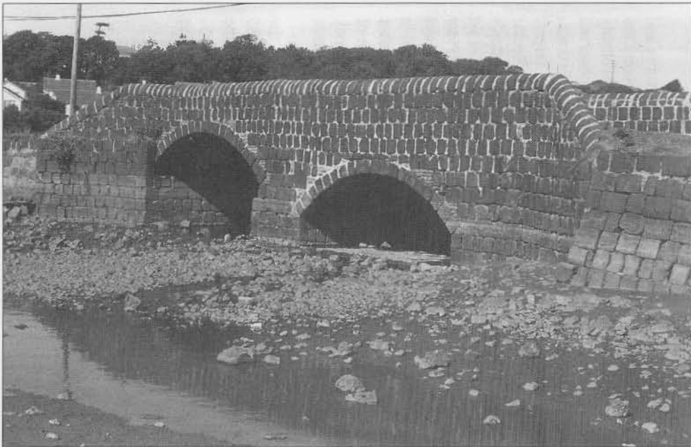
Plate 3. Bridge over Loggans Stream, between Copperhouse and Phillack. Note the height of the arches and batter on right hand revetment.
